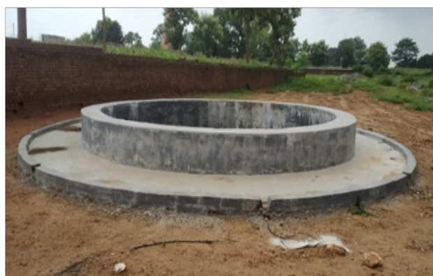
Construction of well at at Sindwar Tand under Marangmarcha Panchayat, CCL Rajrapa
