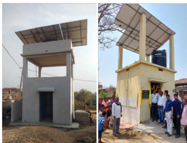
Construction of solar power operated deep borewells with water storage facilities at CCL Magadh-Amrapali and CRS Barkakana
