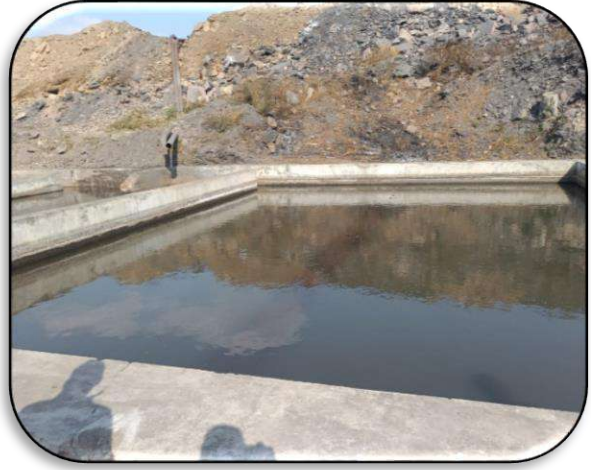
Photo-08 (Settling tank)
