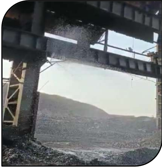
Photo-22 (Fixed Sprinkler at Washery Bunker)
