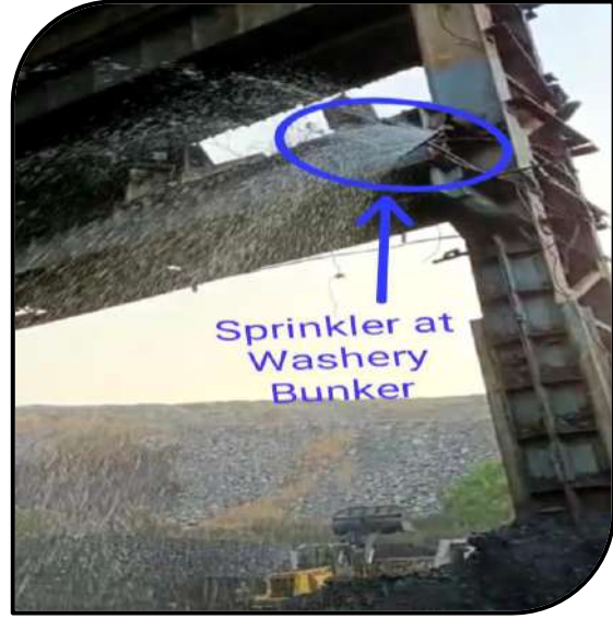
Photo-23 (Fixed Sprinkler at Washery Bunker)
