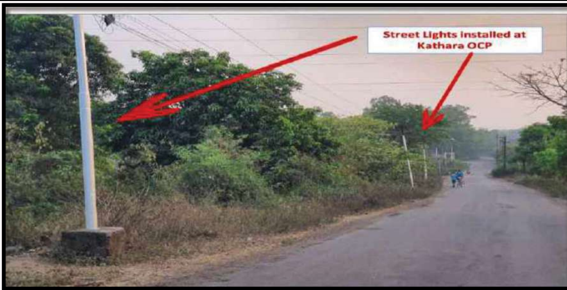
60-watt LED street light installed near Kathara OCP
