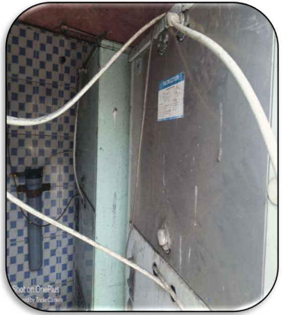
Photo-33 (Aqua guard at pit office for drinking water)
