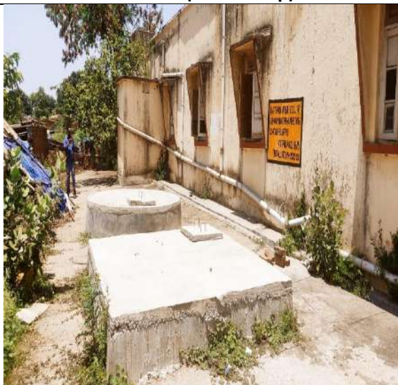
Photo-11 (Rainwater harvesting at PO Office)
