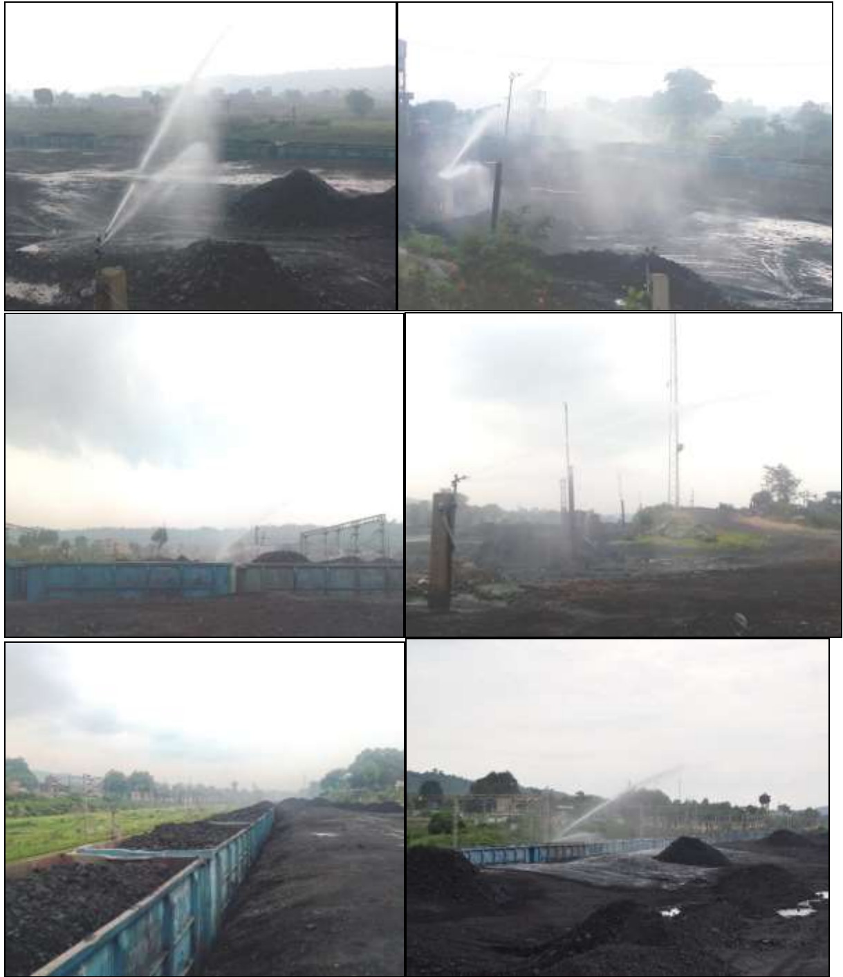
Figure 1.2 High Capacity Fixed water sprinklers on both sides of railway track
