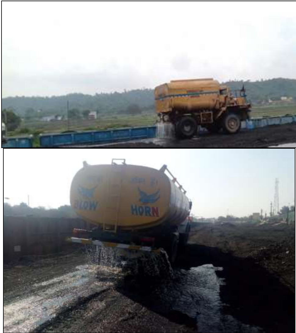
Figure 1.4 28 KL Mobile Sprinkler Mobile water sprinkler at Dakra siding
