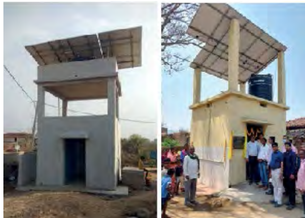
Construction of solar power operated deep borewells with water storage facilities at CCL Magadh-Amrapali and CRS Barkakana
