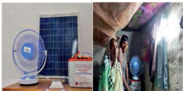
1500 Solar kit installed at a rural house hold of M&A Area.
