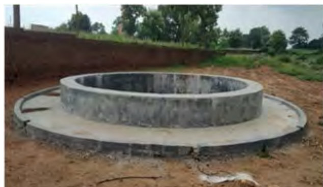
Construction of well at at Sindwar Tand under Marangmarcha Panchayat, CCL Rajrappa
